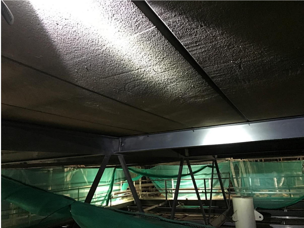
Photo 010 – Sagging RAAC panel.
