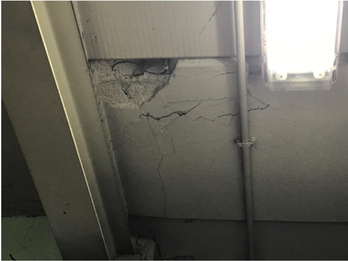
Photo 002 – Damage to RAAC panel.
