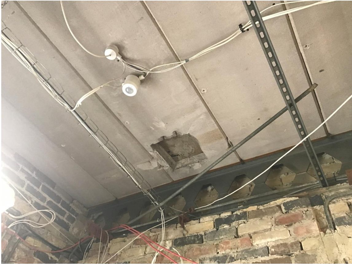
Photo 008 - Damage to RAAC panel.
