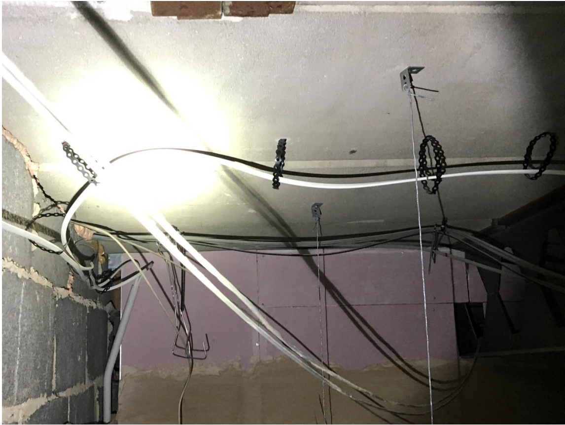
Photo 006 – Sagging RAAC panel.
