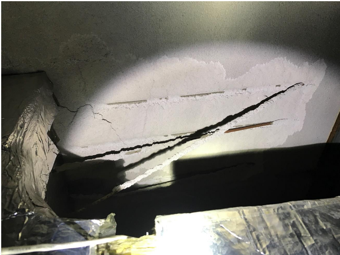
Photo 007 - Damage to RAAC panel, service installation.
