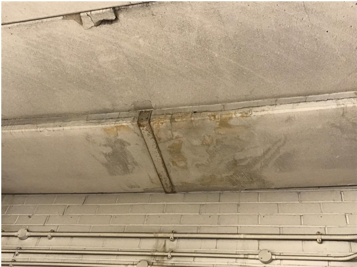
Photo 009 - Sagging RAAC panel and water ingress.
