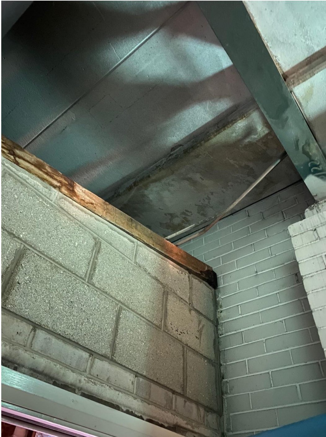
Photo 001 – Water staining and spalling concrete.
