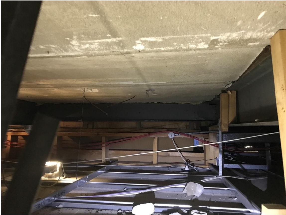
Photo 004 – RAAC resting on suspended ceiling.
