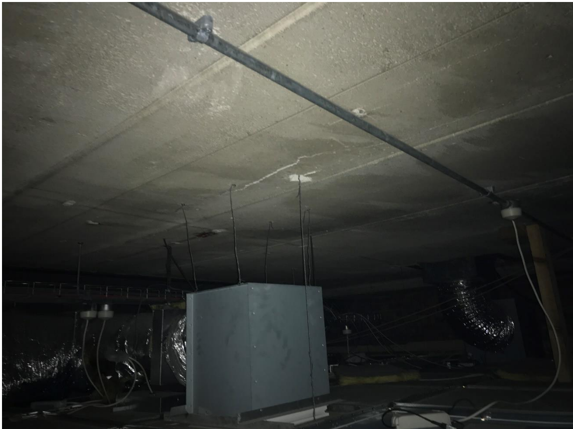
Photo 005 – Distressed RAAC panel.
