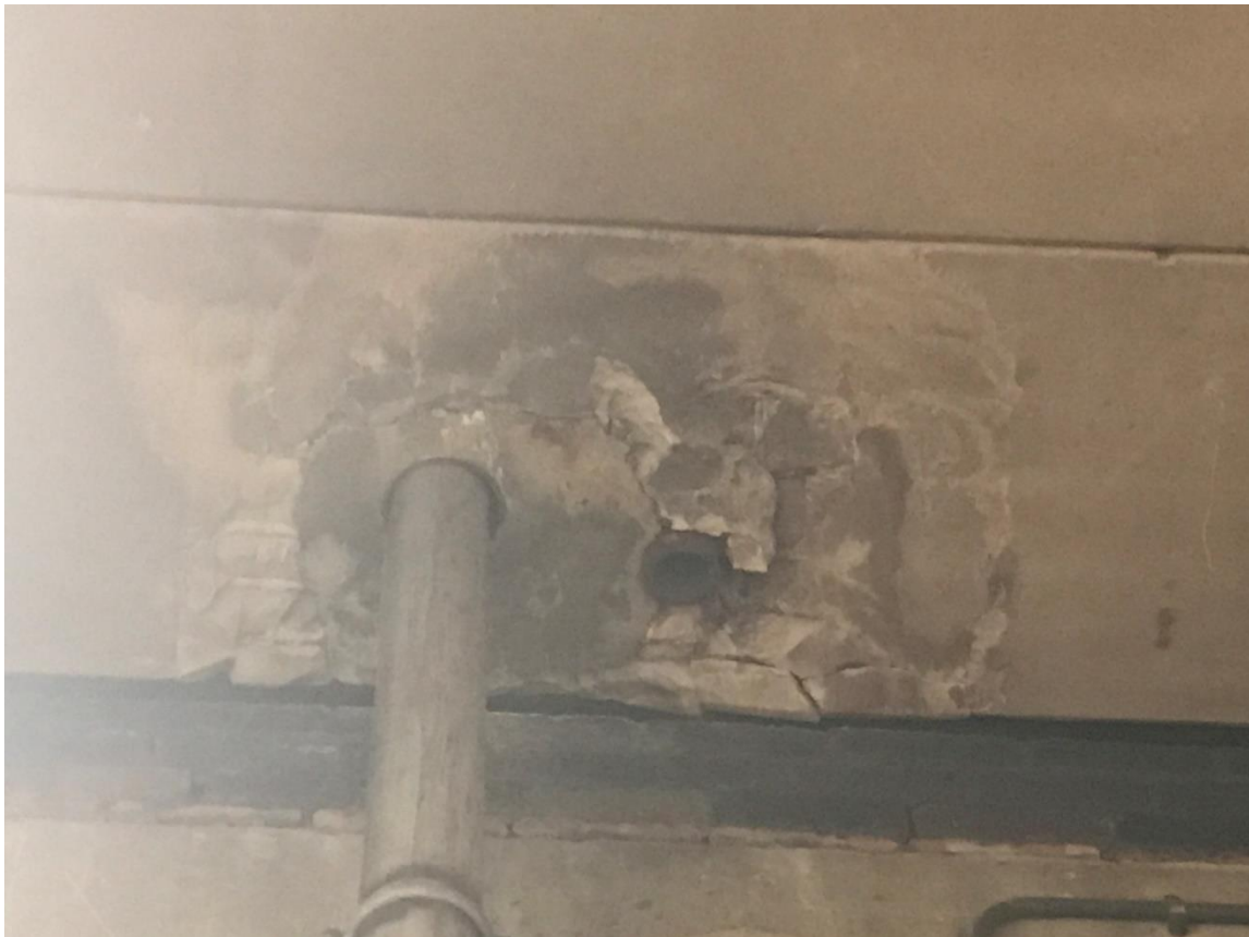
Photo 003 – Damage to RAAC panel, service installation.
